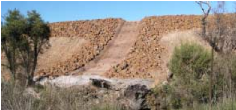
Concave batter slope and spillway, also showing rock armouring of the top (steepest) section of batter slope.
